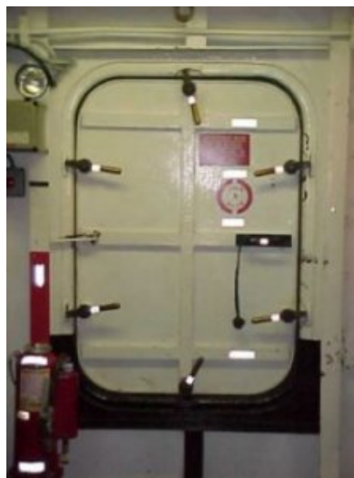
Figure 36. Water-tight Door and Bulkhead From [92]
